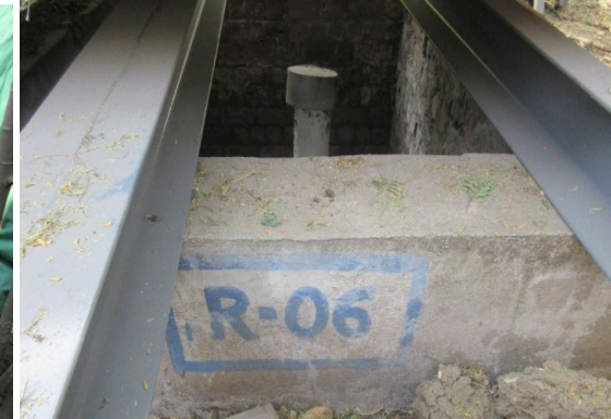
Recharging Pit- 06 Near IBD- XXII
