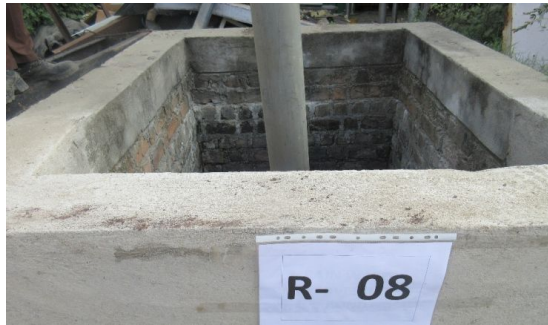
Recharging Pit- 08 Near IBD- XXII
