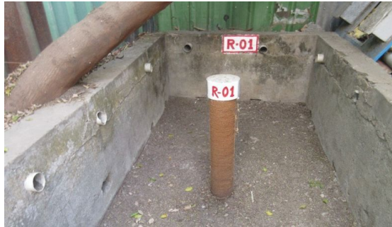
Recharging Pit-01 Near Pharma- I
