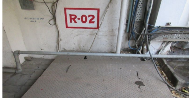
Recharging Pit- 02 Near First Aid
